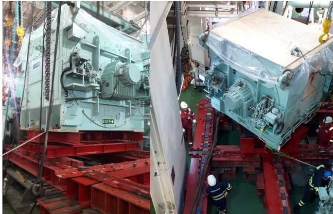
Alternator being skidded along the top of a turning table
